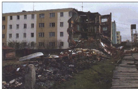
Slip-sliding away. Melting permafrost undercut the foundation of this apartment building in Cherskii, to devastating effect.
