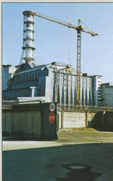
Crumbling sarcophagus. Engineers plan to replace the concrete shell because of concerns about its stability.
