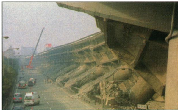
Weak link. Older sections of the Hanshin Expressway between Kobe and Osaka could not withstand the shaking.
