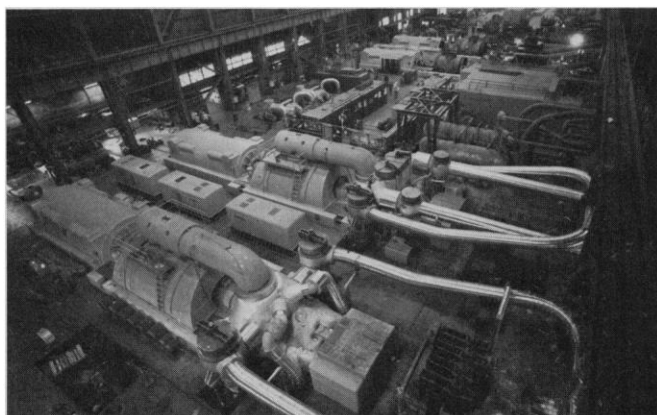
Steam turbine room
