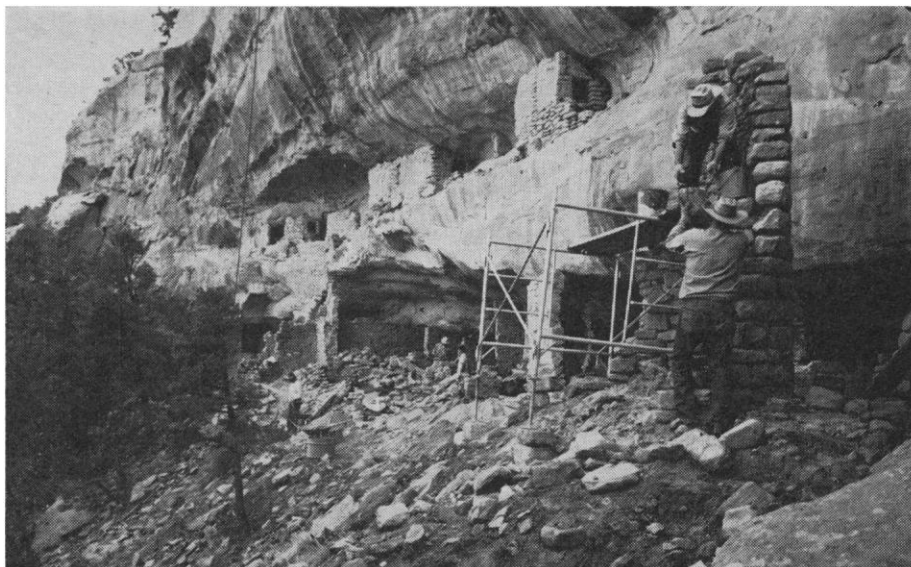
Fig. 6. Stabilization crew at work in a Mesa Verde cliff dwelling. Weak foundations are strengthened, badly preserved walls are rebuilt, and many walls are capped by removing several courses of stones from the tops and edges of walls and resetting them in properly tinted cement.
