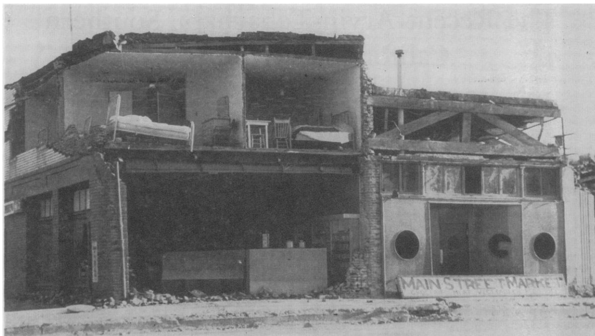
FIG. 1. Earthquake damage in Tehachapi, California, in shock of July 21, 1952. Illustrates a very common type of building failure in earthquakes: toppling outward or collapse of brick parapets, fronts, and side walls, which permits dropping of floors and roof trusses.
