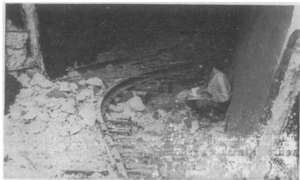
FIG. 8. View into south end of Tunnel 3, showing kinking of track and damage to reinforced concrete tunnel walls, which here were pushed inward over kinked rails.
