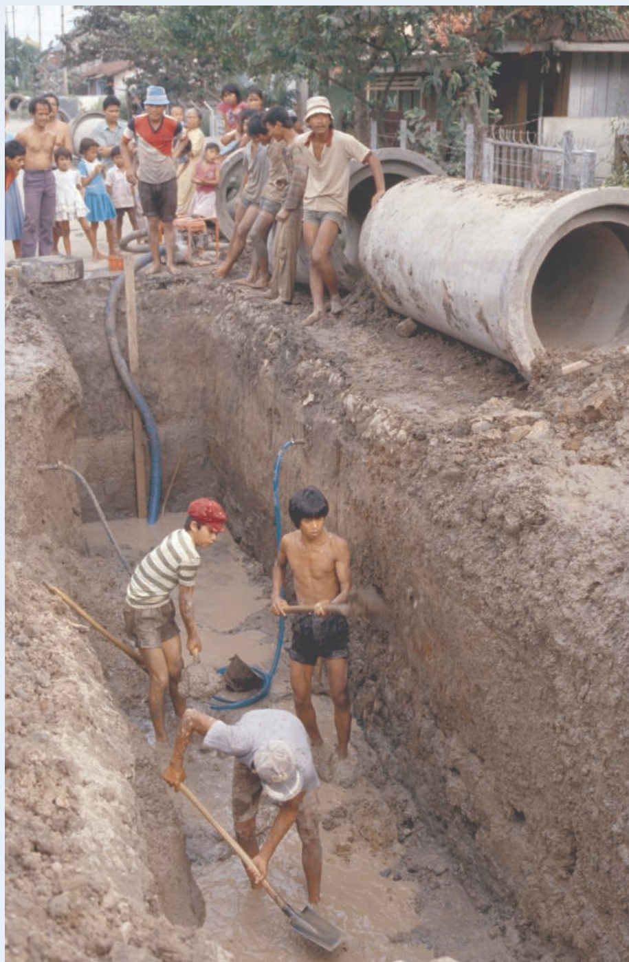
Digging deep. The utility stretched its dollars by installing much of the new distribution system itself.
